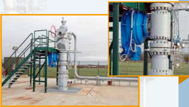
Head of Gas Cavern, VNG AG, Germany
